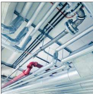
Pipe Freeze Protection
