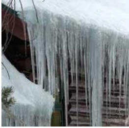
Unprotected roof and gutters
