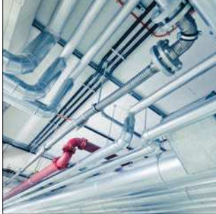
Pipe Freeze Protection
