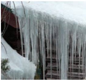
Unprotected roof and gutters
